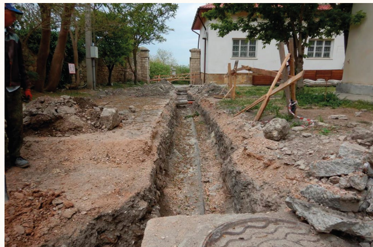
The 45th block. Earthworks for laying utility lines to the buildings transferred to the Monastery. 2024
