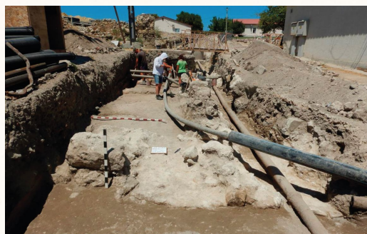
The area of the Southern Gate of Tauric Chersonese. Illegal excavations carried out to free up land for the laying of utility lines to the buildings transferred to the Monastery. Summer 2024.
